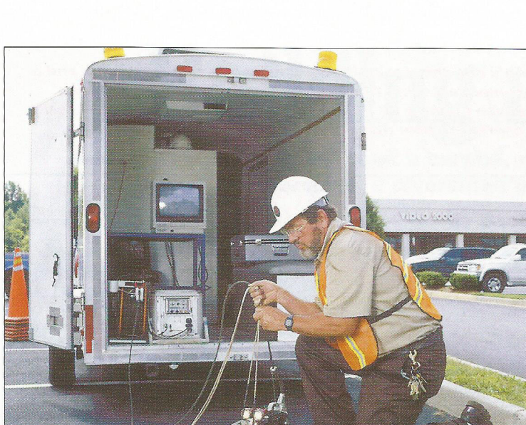
Wayne Norman prepares for an inspection using a Rover crawler. Wayne has built a thriving video-inspection business for Capital City Services.
